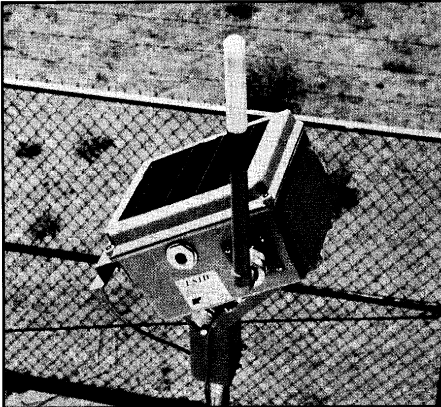
Photo 2-A short-range, electrooptical radiation field sensor is used for preemptive lightning protection
