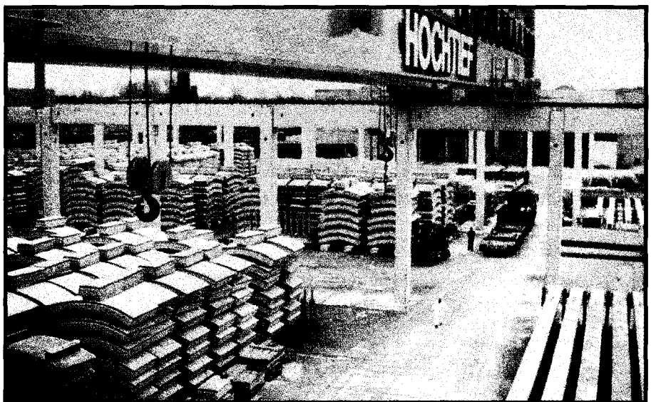
Photo 1—When transporting concrete modules for bridges and tunnels by a crane, sway of the load must be controlled. A fuzzy-logic controller uses the experience of a human crane operator. This crane has two heads, each capable of transporting 64 tons, and it employs an antisway controller based on fuzzy logic.
