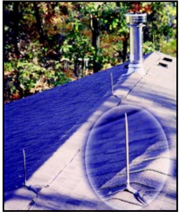
Photo 1 —Any effective lightning system starts with a good array of lightning rods spaced about every 20' along the peak. The insert shows one rod in a little closer detail.
